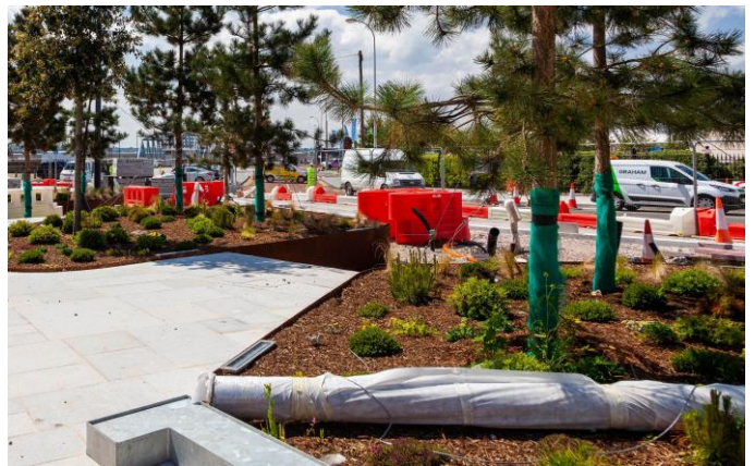
Image above showing the progress of the planters situated at St Nicholas Place
