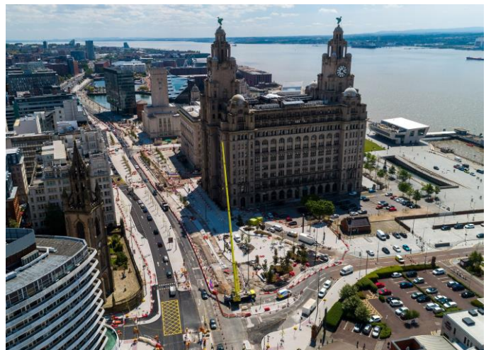
Aerial image showing the completed southbound carriageway surface and St Nicholas Place
